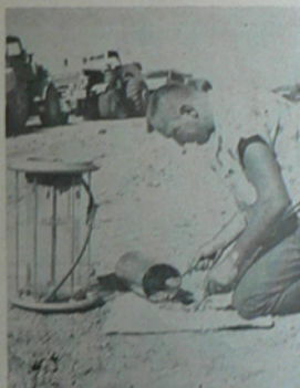
Fred Schabacker checks compacted fill for density determination using water-balloons method at the new City of Phoenix reservoir, a typical step in testing and control by Engineers Testing Laboratories, Inc.
